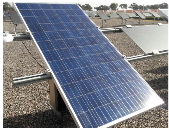
Fig. 3. Outdoor exposed PV panel
