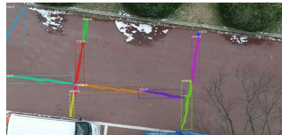
Fig. 4 Example of ideal crack detection (training data set)
