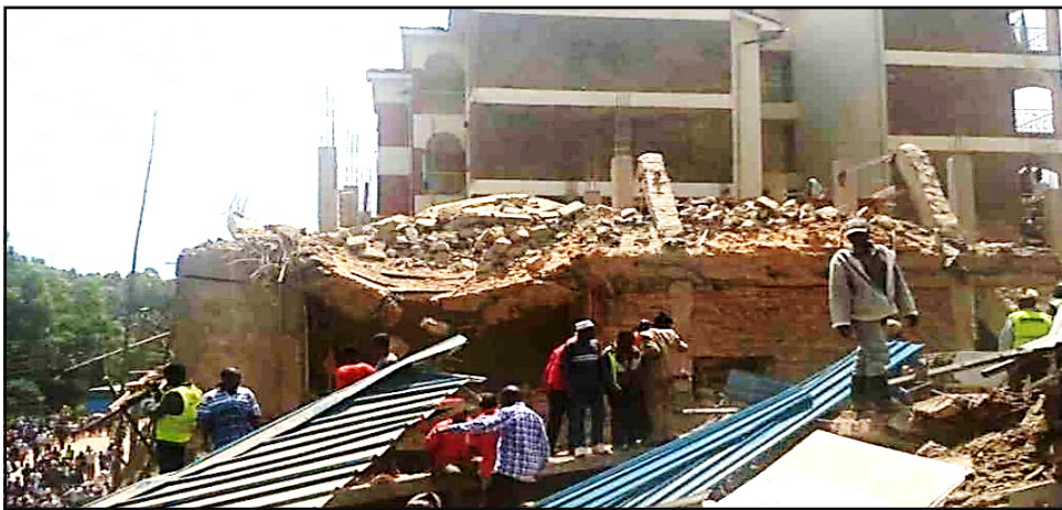
FIGURE III. A BUILDING THAT COLLAPSED IN KISII TOWN
