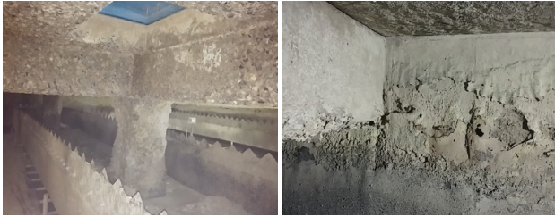
Fig. 1 Deterioration of a structure (delamination from chemical corrosion)
