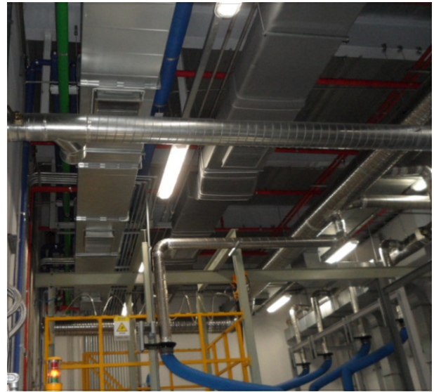
Figure 1. Spray water disturbance by air conditioning duct.
