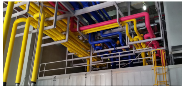
Figure 2. Watering disturbance by utility piping.
