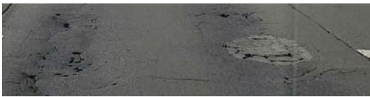
<Fig. 2> Original Image including Road Damaged Area
