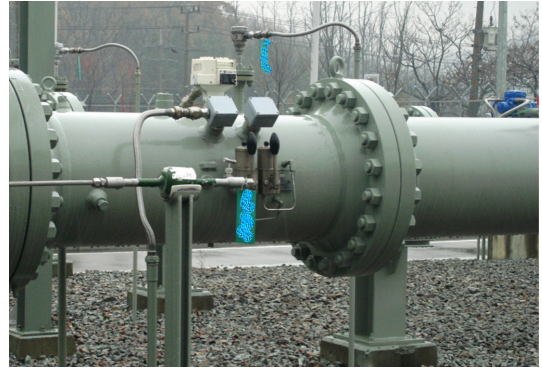
Fig. 1. Example of branch lines attached aboveground high pressure natural gas pipeline in a regulating station.
