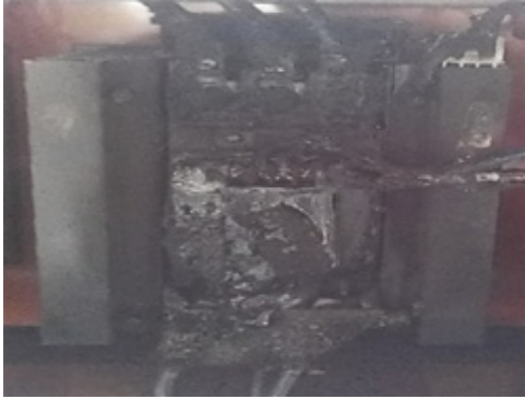
[Figure 8] SSR Fire Field Due to Overheating
