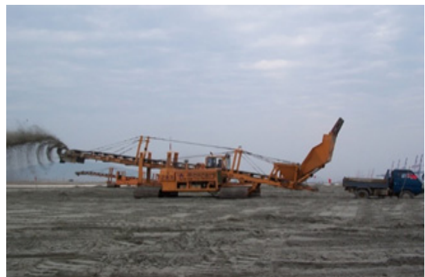
(b) Belt conveyor equipment that covers soft soil with sandy soils (KAITA, 2018)
