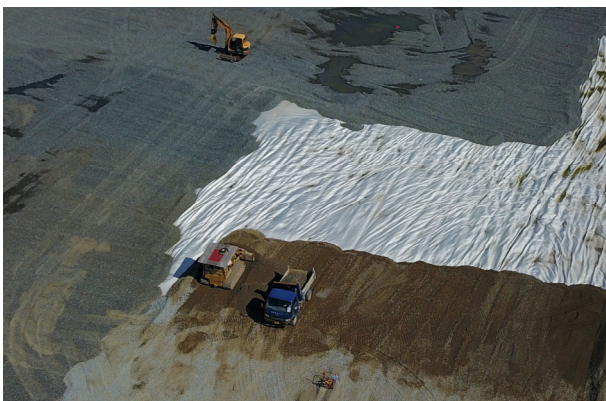
(a) Construction work covering up soft soil with crushed stone and sandy soil (KAITA, 2018)
