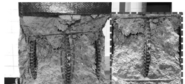
Debonding of the carbon sheet and buckling of longitudinal bars (e) Column C
