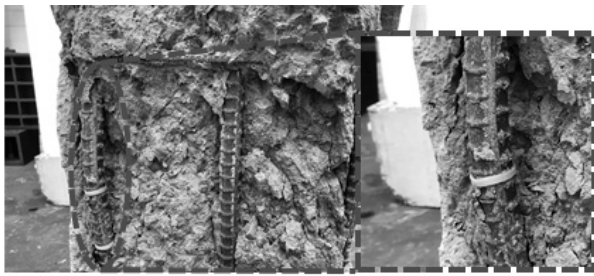
Buckling of longitudinal bars (a) Column E
