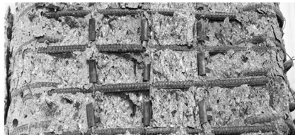
No opening of prefabricated bar unit hoops and U-shape ties (d) Column P
