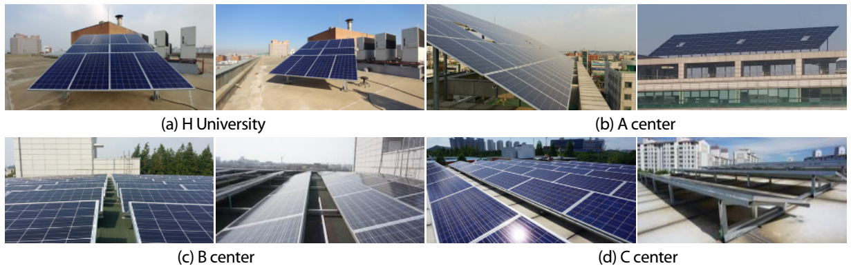
Fig. 3 PV system installation view of 4 sites
