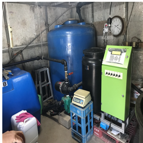
(b) Control panel of hydroponics
