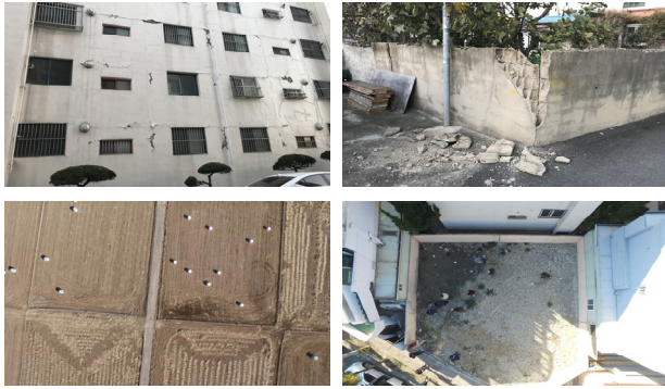
Fig. 3. Damage on site by the Pohang earthquake
