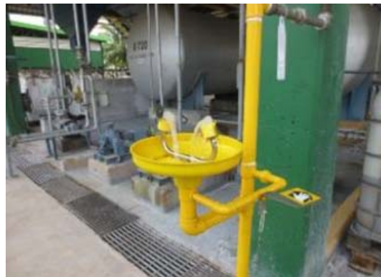
Fig. 5. Inappropriate water height by low pressure
