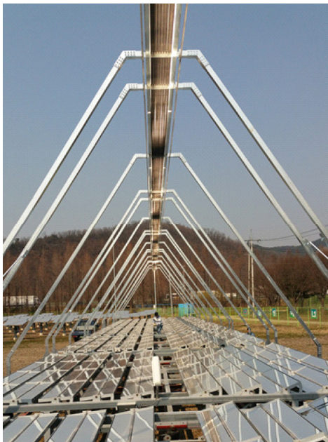
Fig. 5 LFR concentration system
