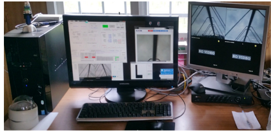
Fig. 6 LFR control system
