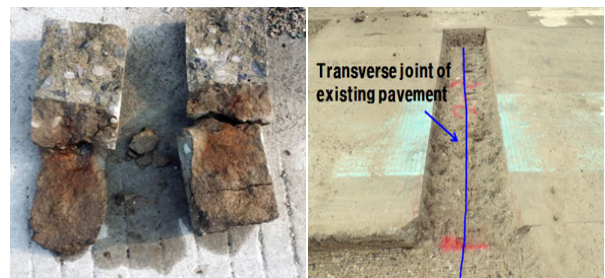
(a) Core Specimen at Transverse Crack (b) Transverse Joint of Existing Pavement
