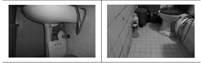
Fig. 8. Risk of dropping a toilet due to aging
