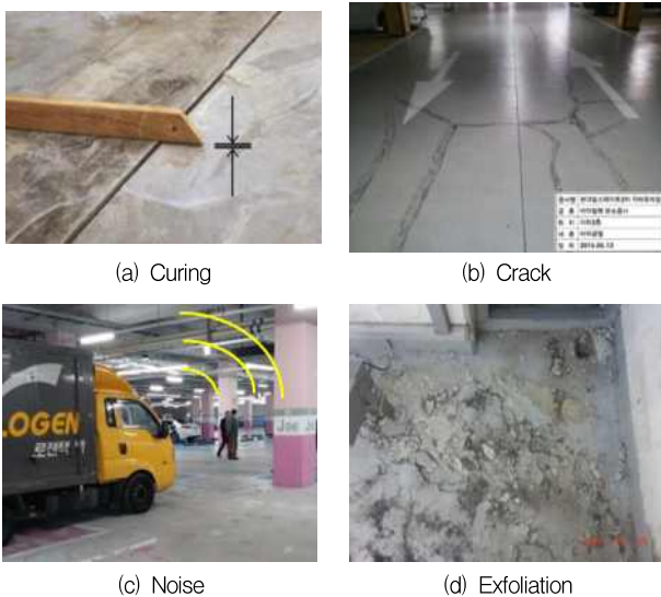
Figure 1. Quality defect of slab plain concrete
