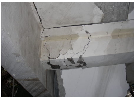
〈Fig. 1〉 Damage of member
