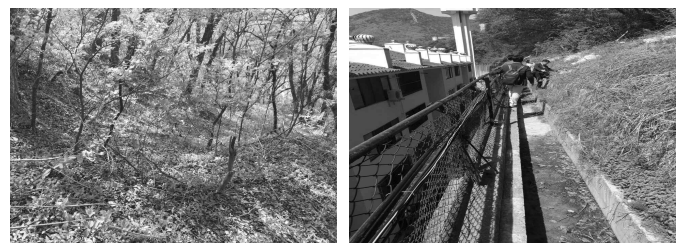
Fig. 6. Water channel formation and defensive fence damage status
