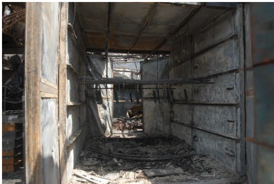
(b) Inside of drying furnace
