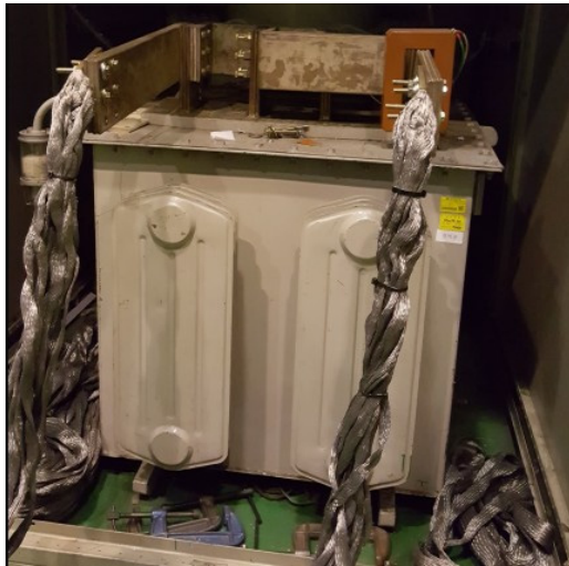
(a) Single phase testing transformer
