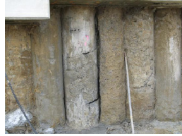
(b) Wall defect due to lack of concrete fluidity
