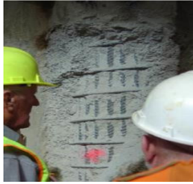
(a) Wall defects caused by dense reinforcement
