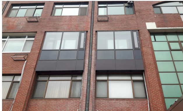
Fig. 4 View of CIGS BIPV curtain wall units applied on an existing building facade
