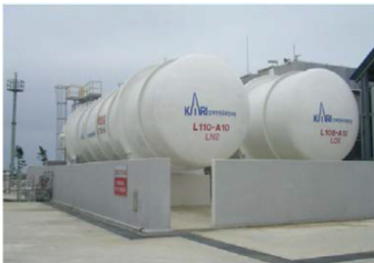
Fig. 3 Photo of liquid nitrogen (L110-A10, left) and liquid oxygen storage tank (L108-A10, right).
