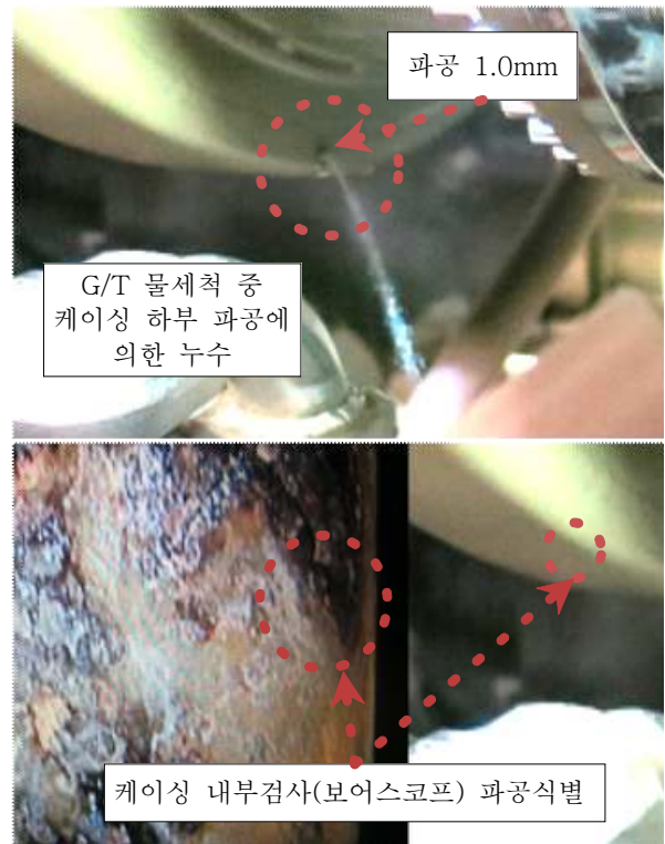
Fig. 9 Damage & Corrosion of G/T Casing[9]
