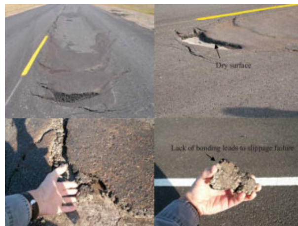
Fig. 3 Premature Failure with Crescent-shaped Cracks after One Day of Traffic (Chen, D., 2010)
