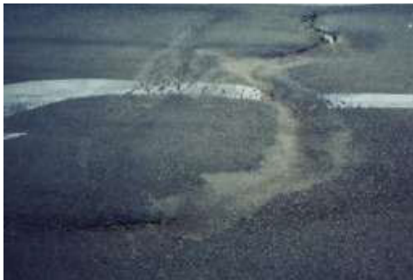
Fig. 4 Asphalt Slippage Failure on Concrete Pavement
