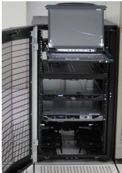
Fig. 6. Server of a central tracking station.
