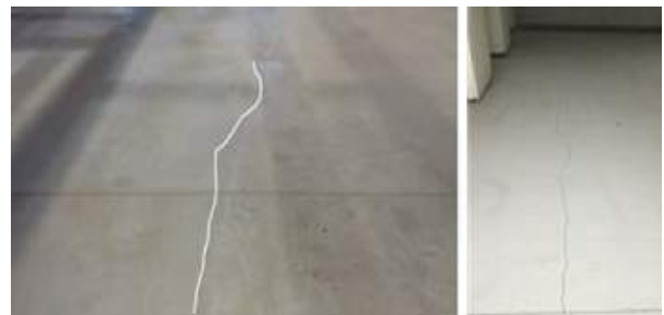
Figure 1. Shrinkage crack on topping concrete
