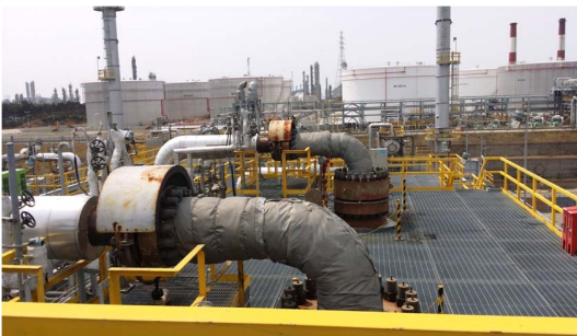
Fig. 7. Topside of Reactor of Residue Desulfurization (RDS) Unit.
