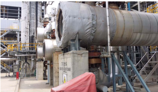
Fig. 6. Heat exchanger of Residue Desulfurization (RDS) Unit.
