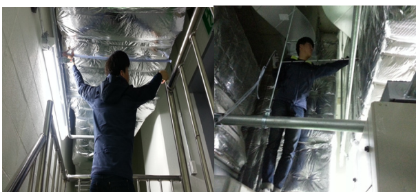
Figure 14. measurement of the duct size, intake and exhaust duct velocity.
