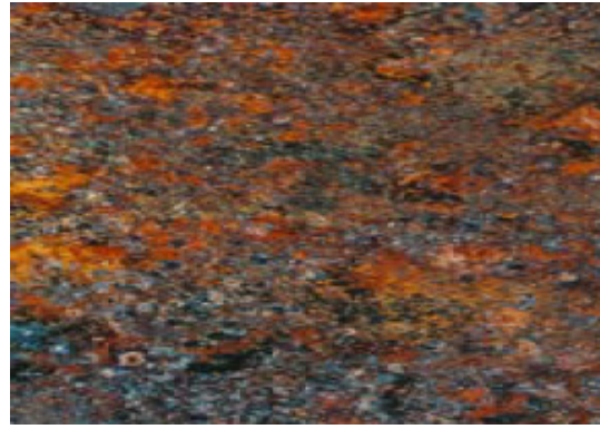
(b) Rust Condition D
