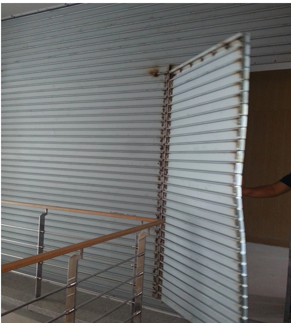
Figure 5. Problem between the integral shutter and stair railings.
