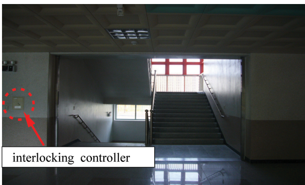
Figure 1. Installed Fire shutter and interlocking system.
