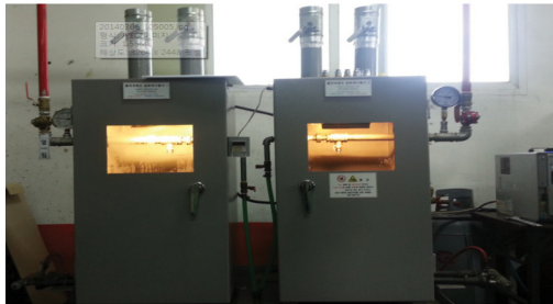
(b) Appearance of the burner
