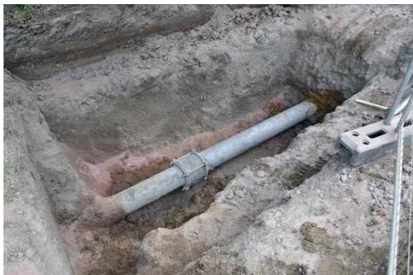
Fig. 1. Cast iron pipe after abrasive blasting.
