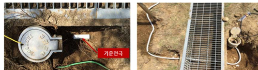
Fig. 8. Installation of reference electrode under T/B.
