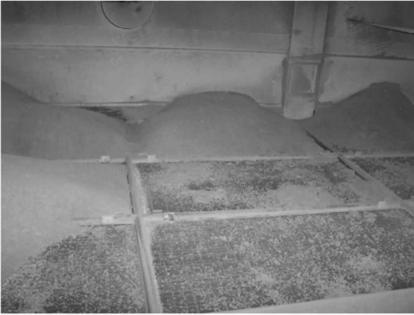
Figure 7. An accumulation of fly ash on SCR catalyst modules.
