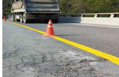
Fig 1. Asphalt road with generated potholes
