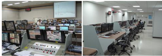
Fig. 2. Launch Control Center(Left), Local Control Room(Right)
