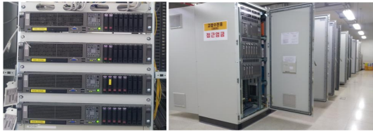
Fig. 3. SCADA Server(Left), Controller(Right)
