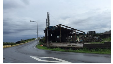
Figure 16. The messy and chaotic construction
