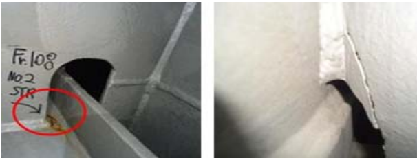
Fig. 8 Fatigue Crack of Slot and Scallop
