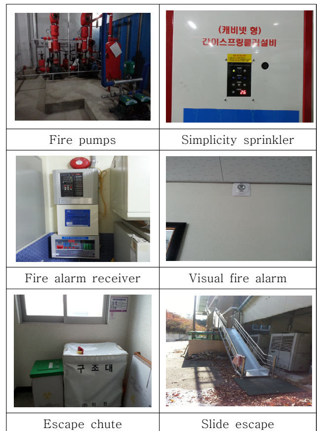
[Figure 2] The pictures of fire safety facility.
