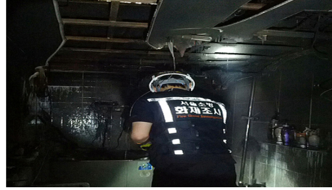
(b) Fire caused by high humidity deterioration
