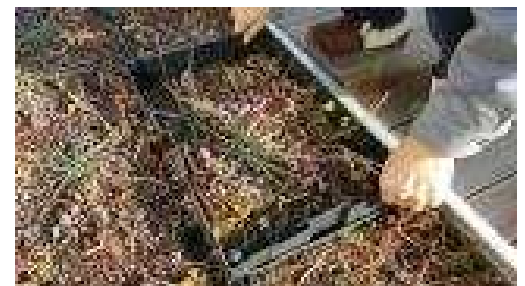
(c) Unit box system with light weight soil and vegetation Figure 6. Materials and unit box system
