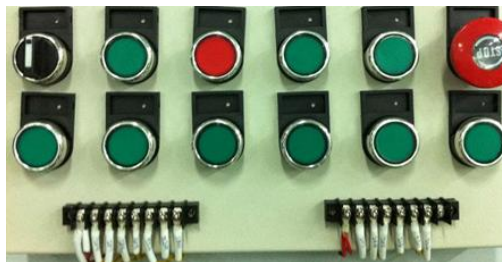
Figure 7. The Control Unit of Photovoltaic Power Generation
