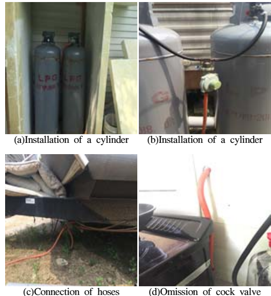
Fig. 1. The insufficient cases of camping facilities.
