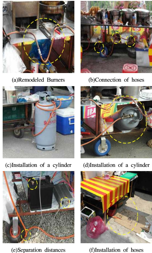
Fig. 1. Insufficient cases of safety management of gas facilities.
