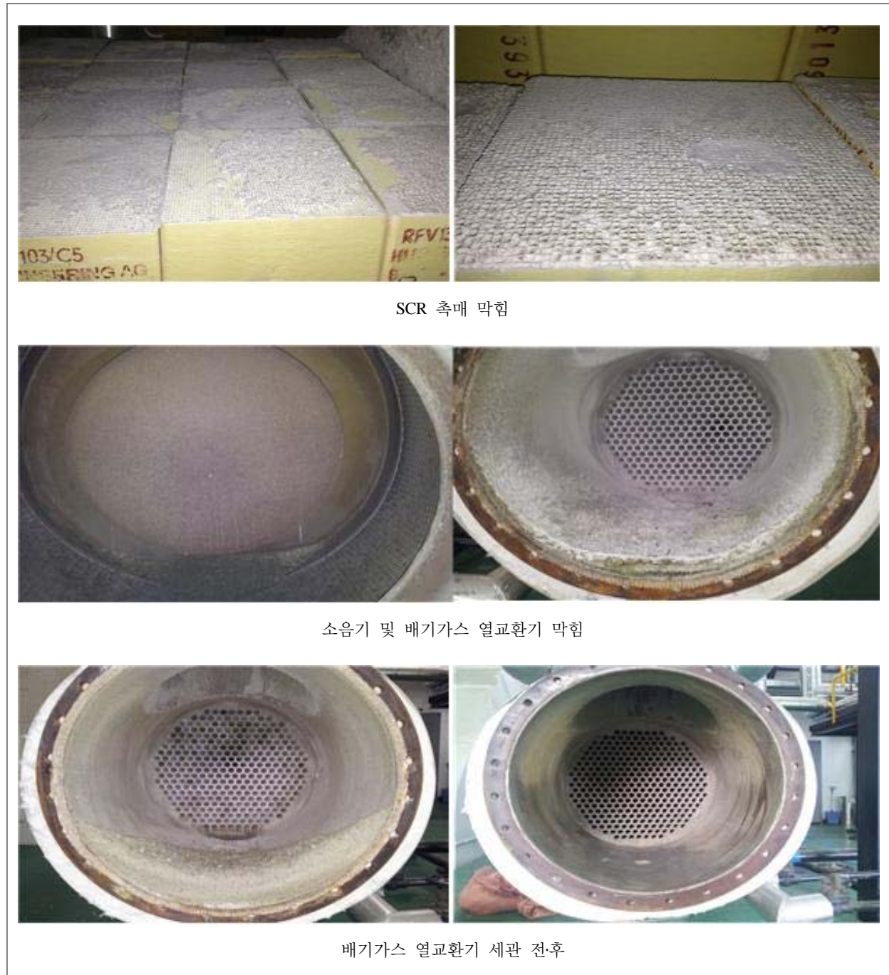
Fig. 3. SCR \Delta P increase and Exhaust gas heat exchanger and silencer clogging case
