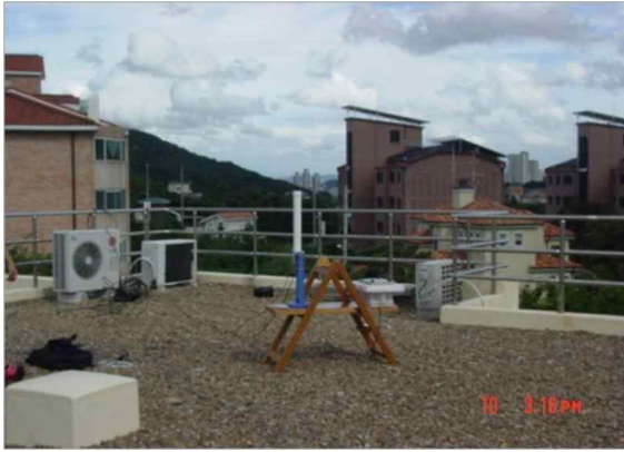
Fig. 7 Antennas on the roof of National Maritime PNT Office
