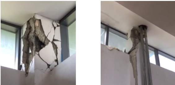
Fig. 13. Short column shear failures during Gyeong-ju earthquakes (2016)
